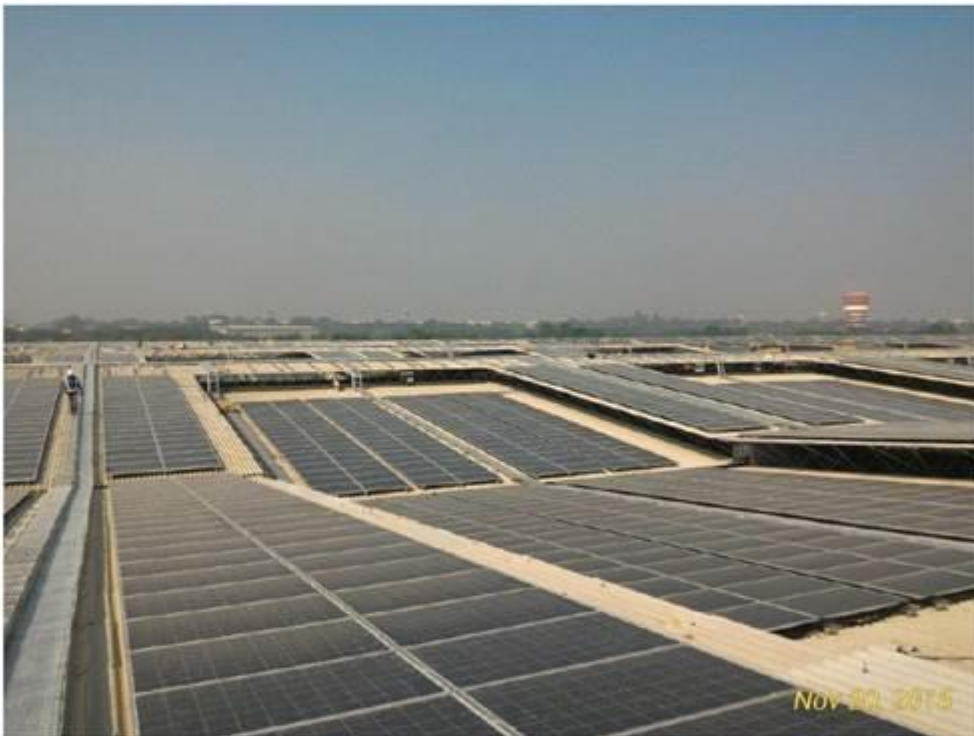
Radhaswami Satsang – 12MWp
